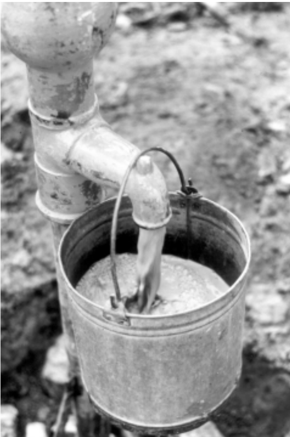
Figure 9.2 Borehole inadequately developed and left for user to sort out
