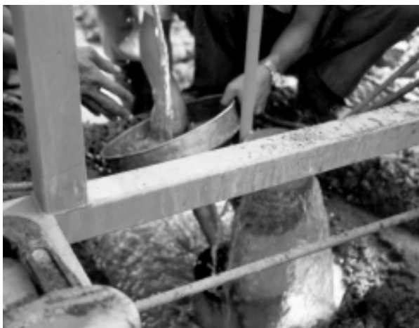
Figure 7.18 Gravel packing being added by funnel note water overflowing casing – gravel dropping below screened layer
