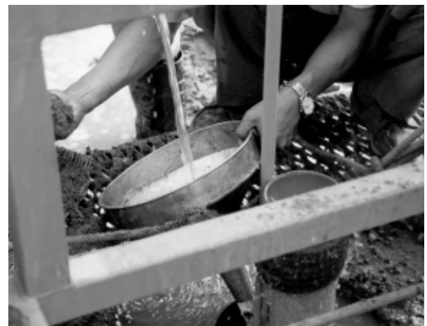
Figure 7.19 Gravel packing – note water flow up has stopped – gravel landed above screen level
